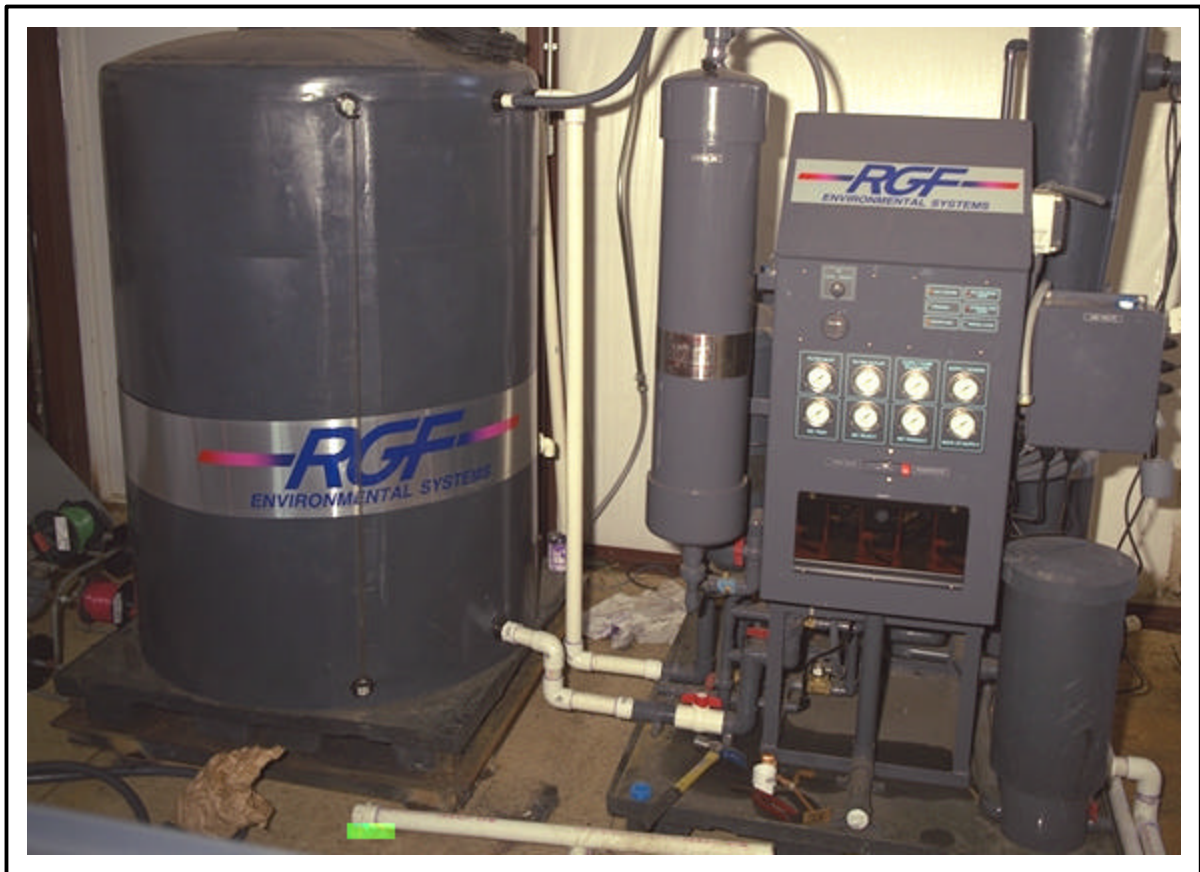
Figure 3. RGF system in Building 338 washrack, Aberdeen Test Center.
